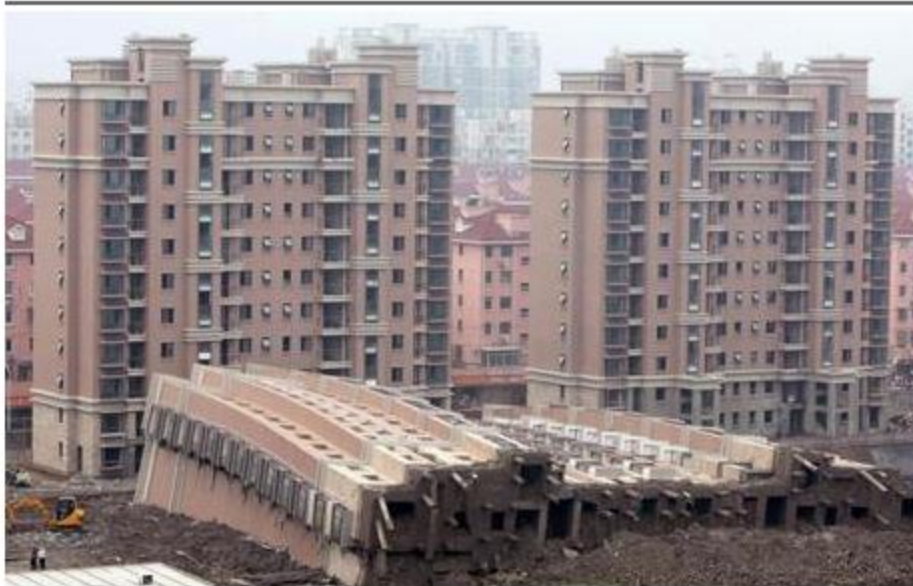
A general view of a toppled 13-storey apartment building that buried one worker in Shanghai. Photo: Reuters
